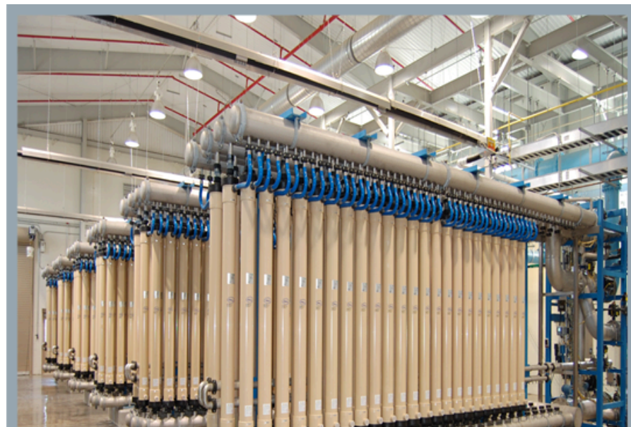
Membrane Filtration System
